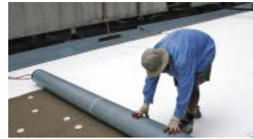
Green Roofing Experts: GAF
